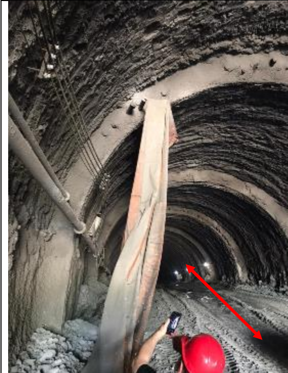
Accident location N7 Entrance of the Tunnel
